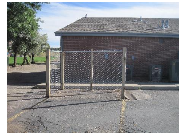
Deteriorated/substandard enclosure, deteriorated pavement, lack of access to public street (Factors a , c and e )
