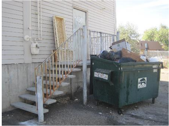
Deteriorated external finishes (Factor a)
