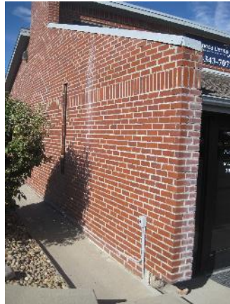
Deteriorated external finishes, poor drainage (Factors a and d)
