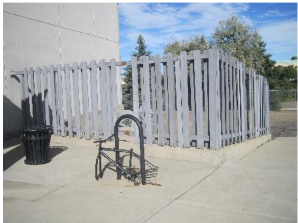
Deteriorated enclosure, abandoned bicycle (Factors a and d)
