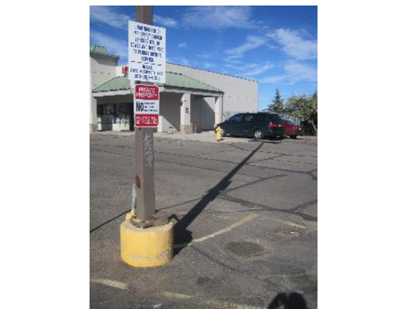
Poor internal circulation, substandard drainage/landscaping, deteriorated pavement, graffiti (Factors b , d and e )
