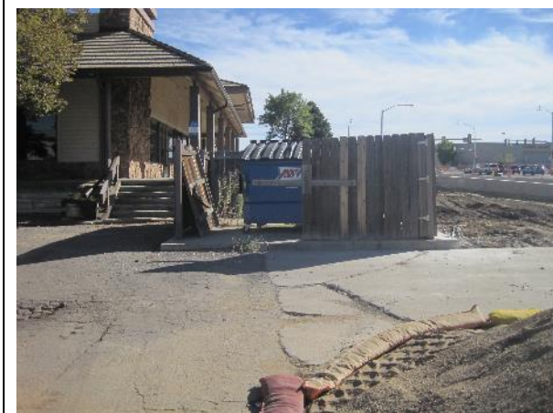
Deteriorated enclosure, loss of access to Sable Boulevard, deteriorated pavement (Factors a , b and e )
