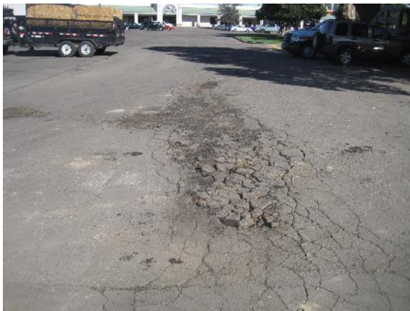
Deteriorated site pavement (Factor e)
