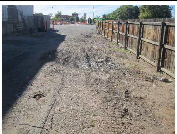
Deteriorated/lack of pavement (Factor e )
