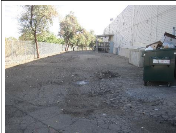
Deteriorated pavement, substandard landscaping, graffiti deteriorated utilities (Factors d and e )
